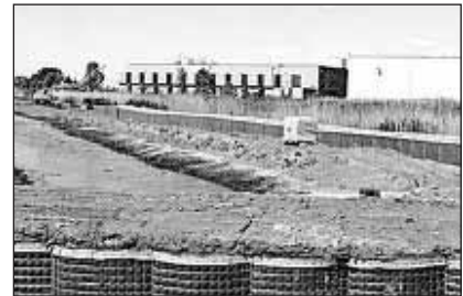
New berms will both channel water into wetlands and protect nearby property from flooding.
